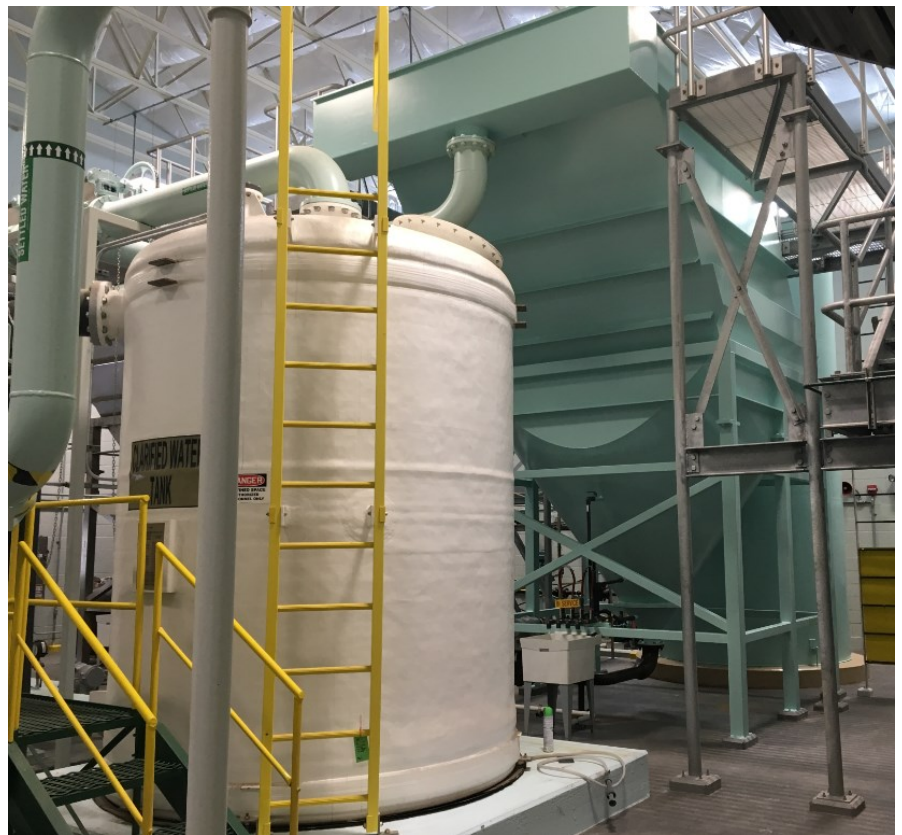
Parallel Plate Clarifier
