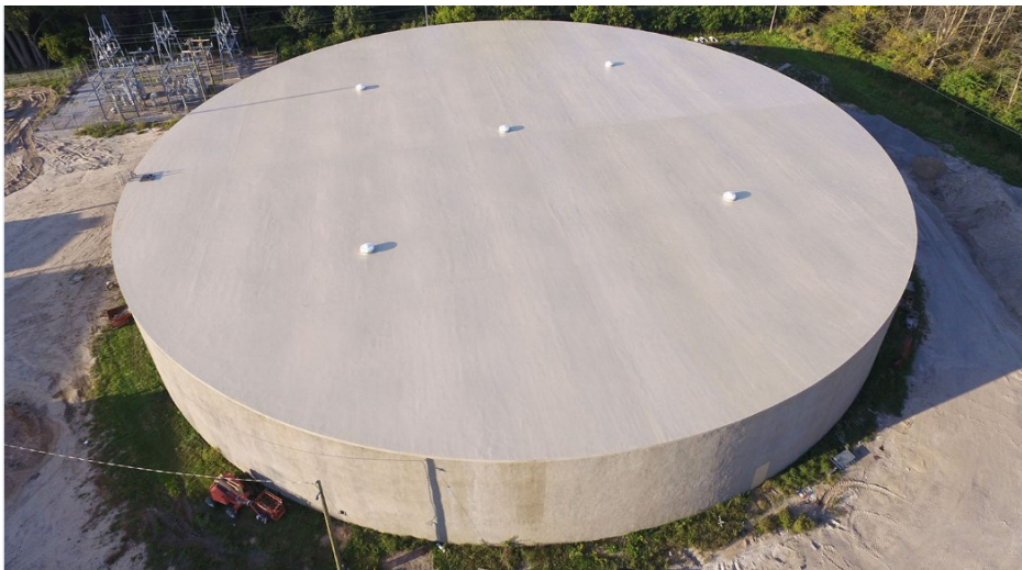
10 Million Gallon Raw Water Storage Tank
